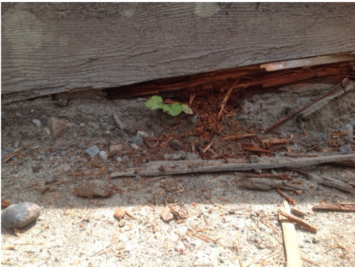
riser rot - only on ones with sediment accumulations on
